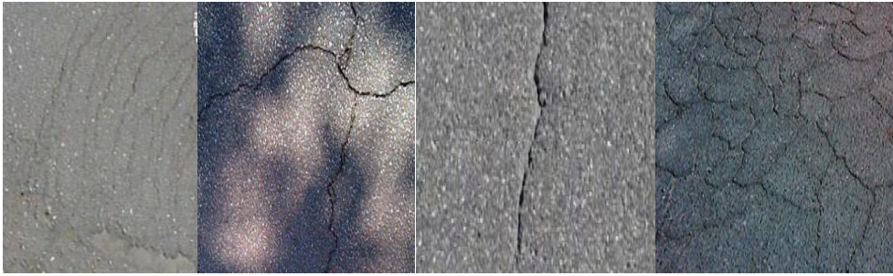
Fig. 3. Four types of cracks: (a) scattered cracks, (b) network cracks, (c) obscure cracks, (d) fine cracks.
